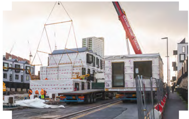
Modular homes produced off-site can significantly reduce the embodied carbon of a project | New Islington, Manchester
