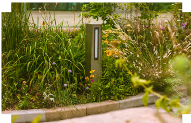
Subtly integrated bollard lighting along green pedestrian route | Charter Square, Sheffield
